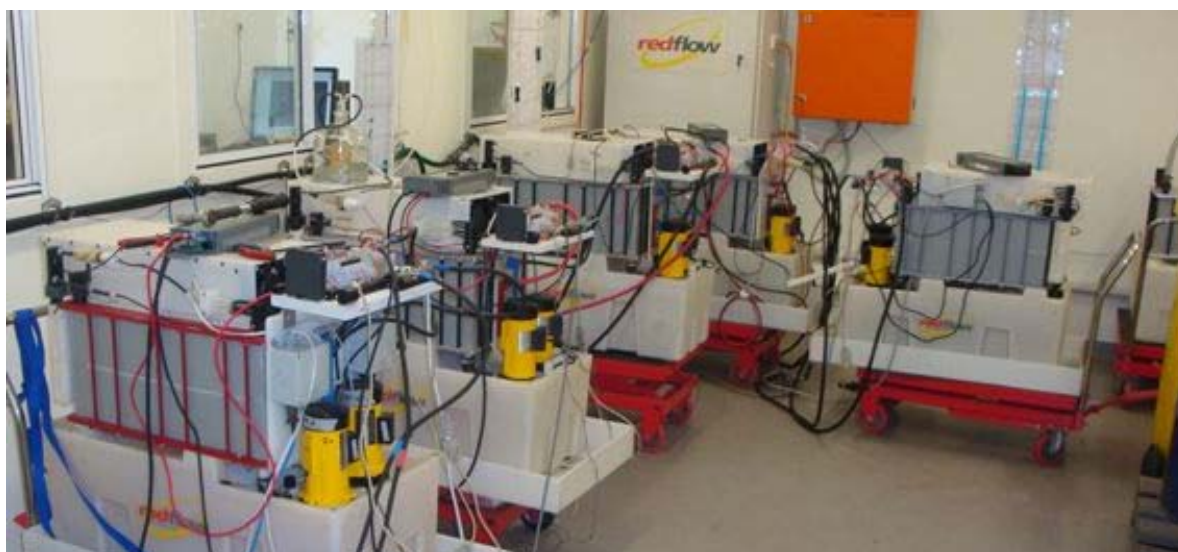
Zinc-bromine batteries undergoing test at RedFlow plant, August 2009
