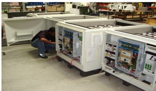
Systems being assembled for the Karara SWER project
