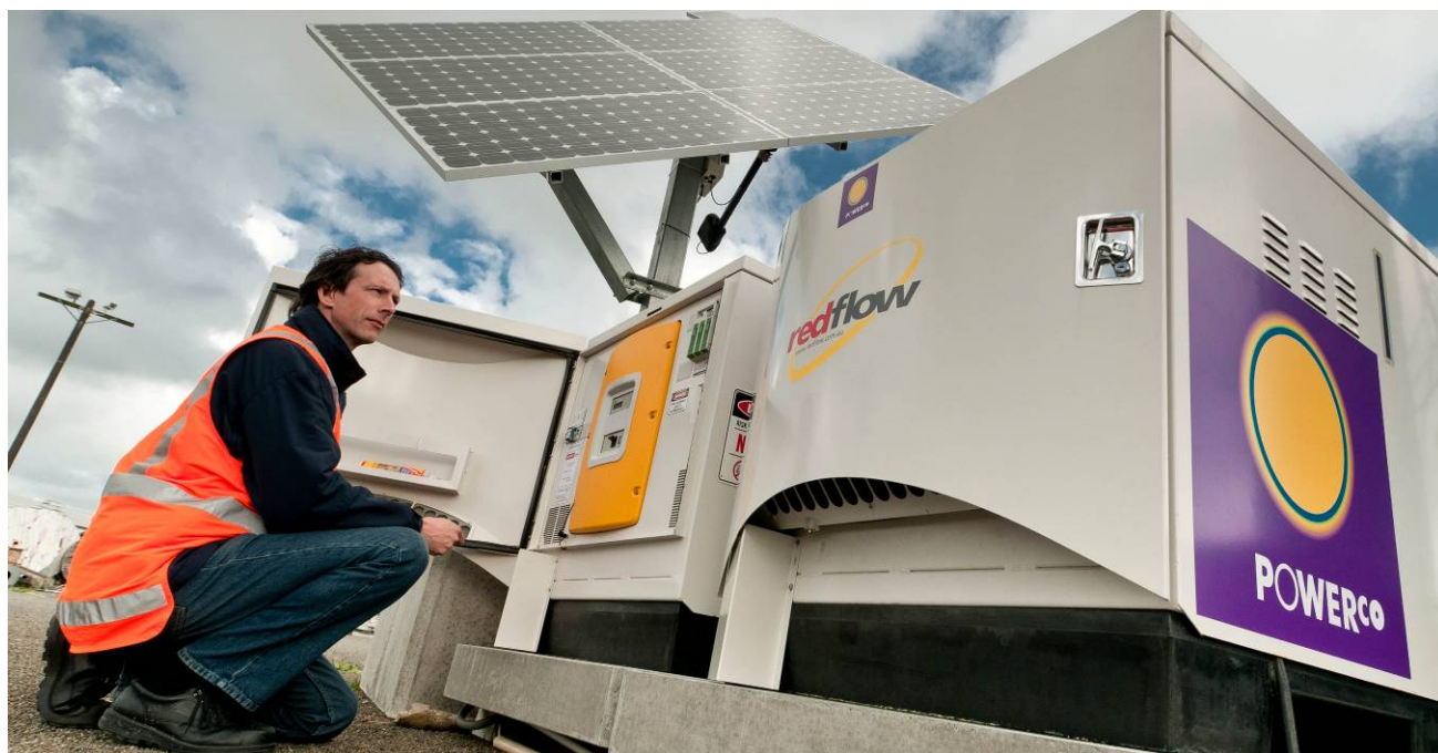
A RedFlow system combined with solar PV panels on demonstration at Powerco's depot in Palmerston North, New Zealand
