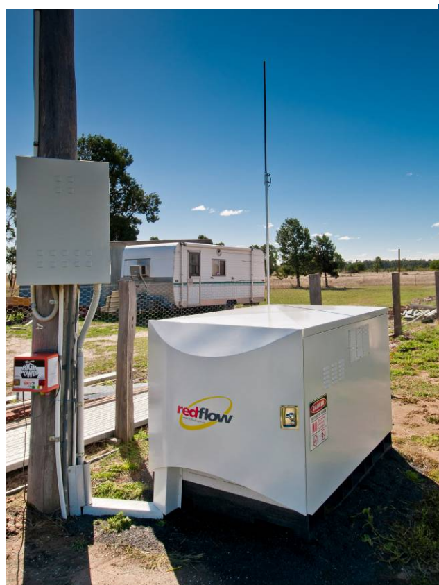
A RedFlow 5 packaged energy storage system at work within the Ergon energy network.
