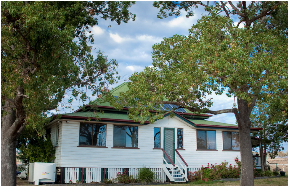
A Power+BOS® energy storage system working at a rural Queensland location. This delivers electricity generated from solar PV in the daytime during evening peak demand times.
